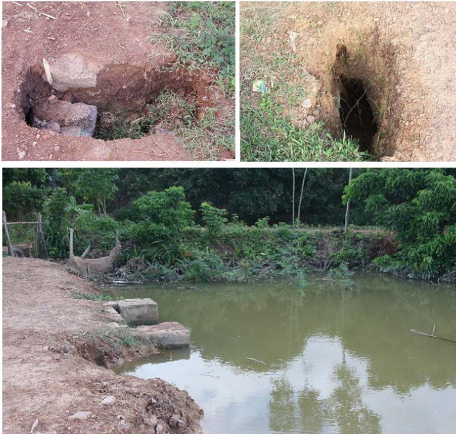
Figure 6 Piping failures resulting from construction or material defects and inappropriately designed spillway
